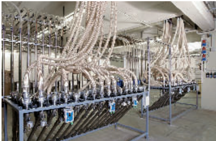
Manual coupling station with decoded device
