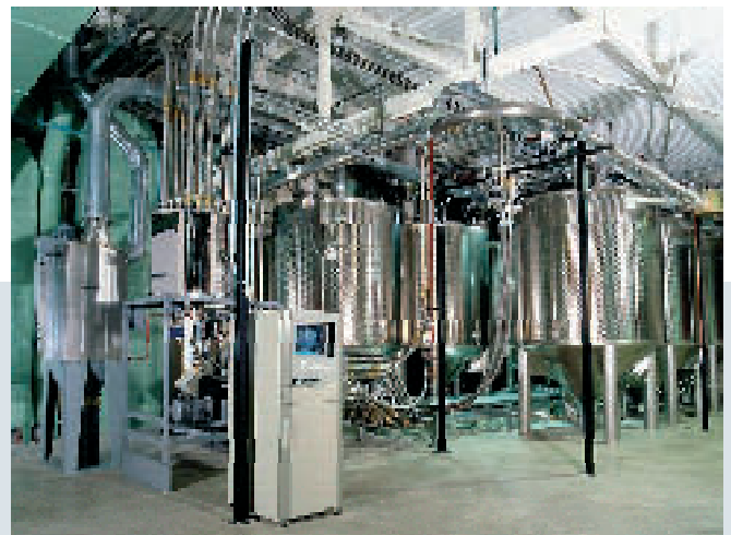
Storage area with automatic coupling station and supervisory system
