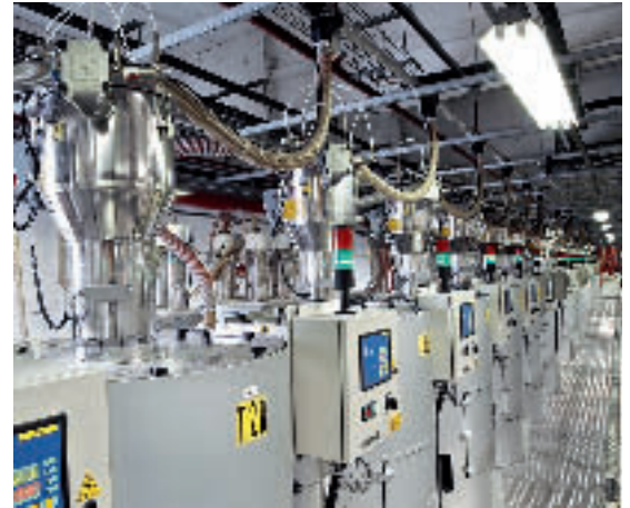
Easy 2 System vacuum receivers for the drying and dosing area
