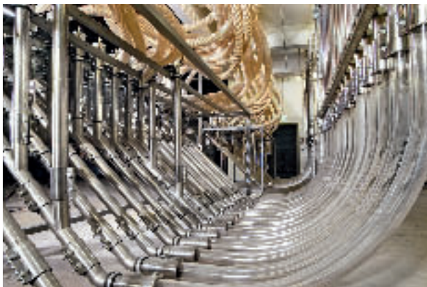
Coupling station with glass bends
