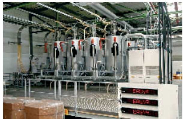
Display signalling the functioning of the conveying system
