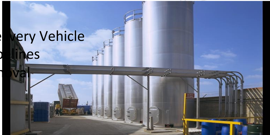
Delivery to One of Six Fifty Tonne Silos
