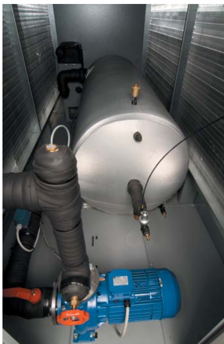
Internal tank with relief valve and make-up valve. Internal pump. Stand-by pump ready
